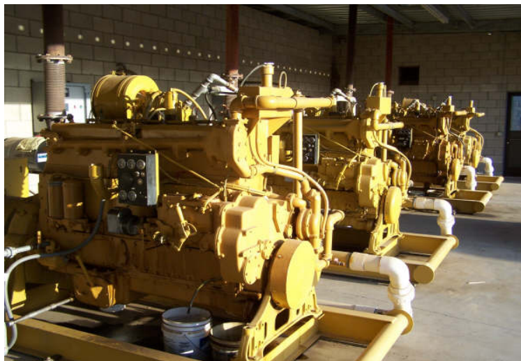
The methane-run generators at Hilarides Dairy.
